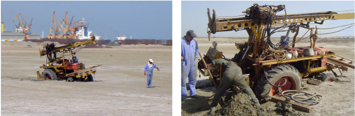
Figure 6- Investigation truck is trapped due to the loose ground conditions in dredging material
